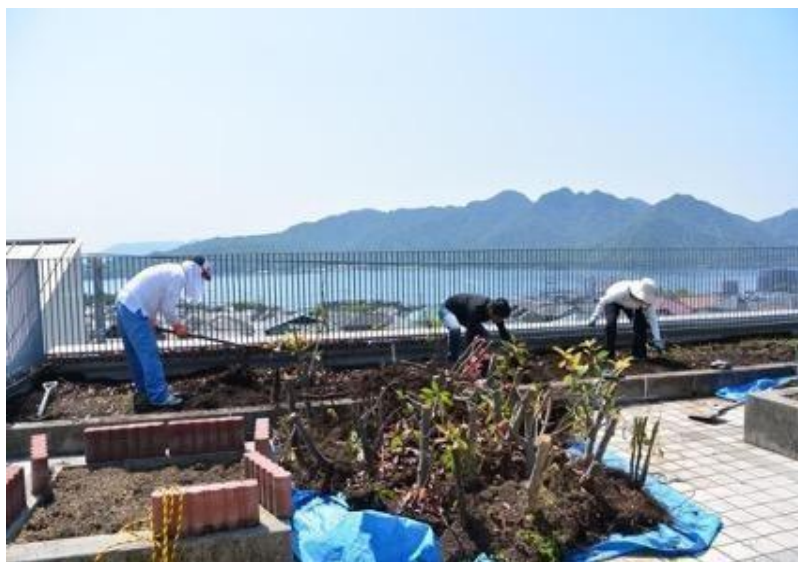
Fig. 8: Site clearing to achieve a beautiful view of the Sato Inland Sea and Miyajima Island from the rooftop garden: 'Therapeutic Sensory Stimulation Garden'.
