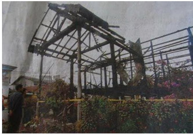
Fig. 2: Rumah Pak Ali was destroyed in a fire on 20 October 2003 (Source: http://fireheritage.blogspot.com/ )
