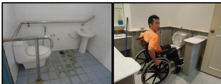
Figure 14 & 15: Accessible toilet is provided but the design and specifications are not according to MS 2015: PART 1: 2006 making the purpose of providing accessible toilet is useless.
