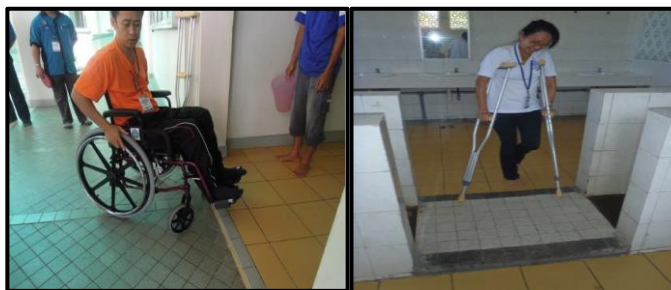
Figure 12 & 13: Entrance to the ablution area and toilet has split levels and some Mosque has design of threshold that is a total barrier.
