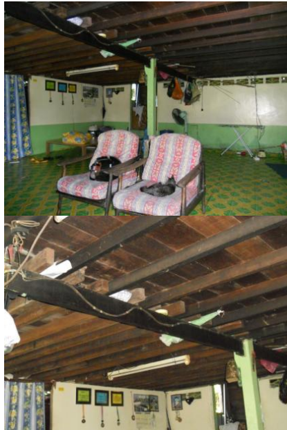
Figure 14: Interior of a villager's house on ground floor. The space between floor joists use for storage Source: Author
