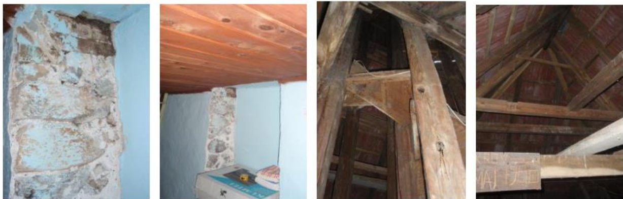
Fig. 3: Brezovača mosque condition of the wall and roof beams in 2017
