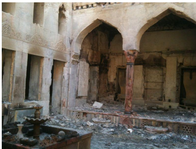
Figure 14: Destruction of Zamria courtyard, Zamaria.com
