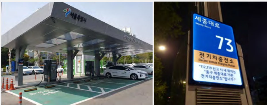
Figure 11: Seoul EV Charging Stations
