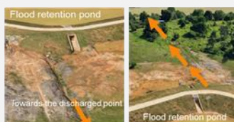
Figure 5: Lack of proper drainage for waterflow from flood retention point to discharged point
