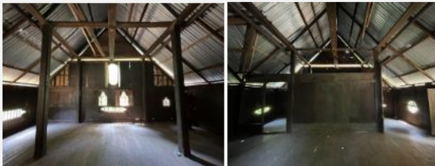
Figure 9: Current condition of rumah ibu
