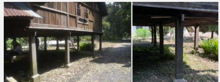
Figure 8: Current condition of the pillars of Rumah Kutai Tok Saudara Bongsu
