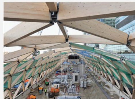
Figure 8 : Timber roof under construction. Galvanised tubes that will supply air to pillows are visible from this angle, but were carefully positioned so they cannot be seen from eye level. Concrete floor forms roof to retail units below, prior to receiving waterproof membrane and soil for garden
