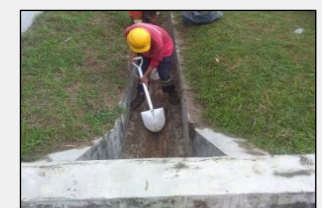
Figure 14.1: Main drainage cleaning program
