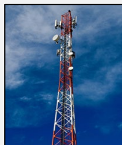
Figure 4.8.1: Example of telecommunication tower (Source: Google Image)
