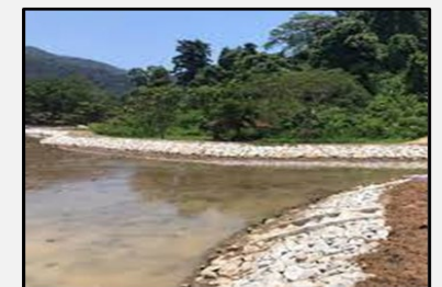
Figure 4.7.2 Example of flood barriers built on the riverbanks (Source: Fieldwork).
