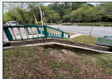
Figure 16. Lack of safety barrier on site. (Source: Author, 2025)
