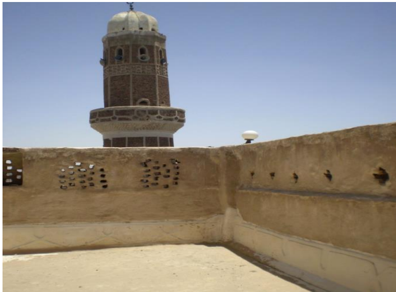
A well protected open roof by a parapet in a house in San'a, Yemen.
