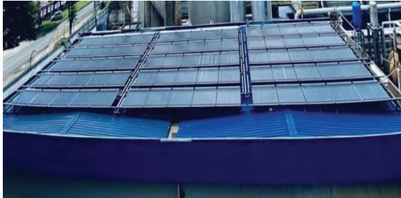
Fig. 1: Array of Evacuated Tube Collectors (front view).
