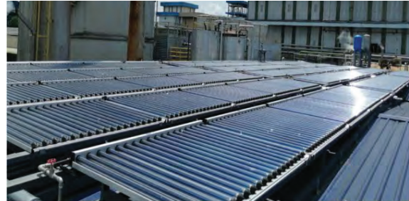
Fig. 2: Array of Evacuated Tube Collectors (side view with 10 degree inclination).
